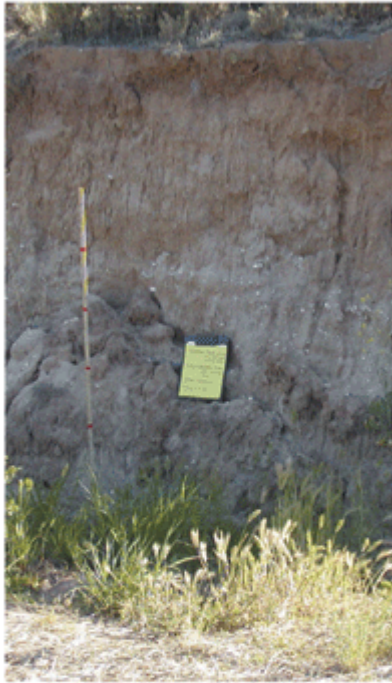
Historically, this road cut (approximately seven-feet deep) eroded during the rainy season, depositing several feet of soil onto a nearby vineyard that had to be manually removed each year. BMP implementation included grading and planting of barley and fescues to reduce erosion and stabilize the area. (Photo by Dawn Stimson)
